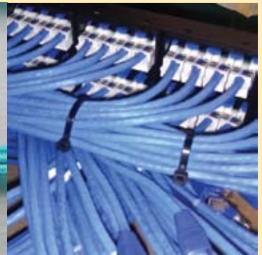
Ethernet & "Rack and Stack" Servers
