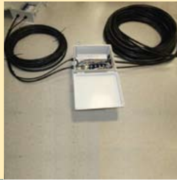
Fiber to the Antenna
